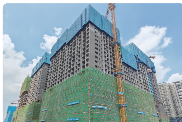
项目采用了装配式外墙、ALC隔墙板、叠合楼板等装配式工艺
